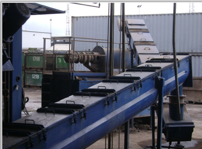
Figure 2: Thermal desorption unit feed system
